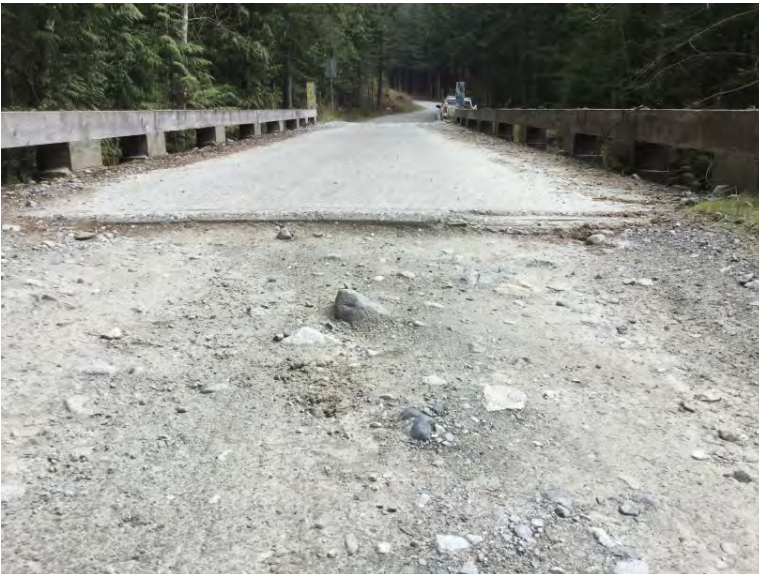
Requires surfacing at both approaches
