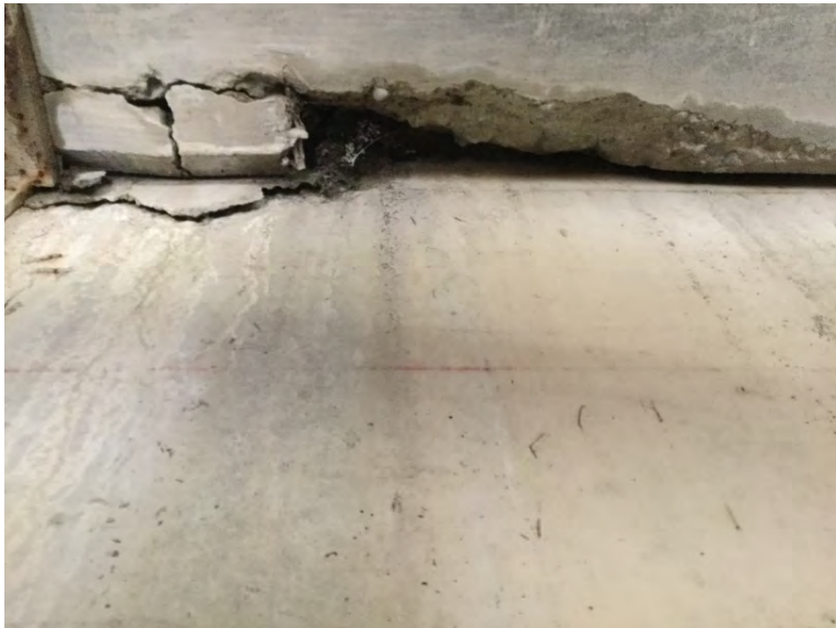
Right bank panel 1 damage
