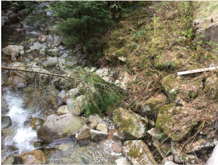
Riprap scour noted downstream right bank
