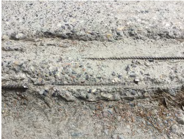
Missing rebar on right bank ballast wall
